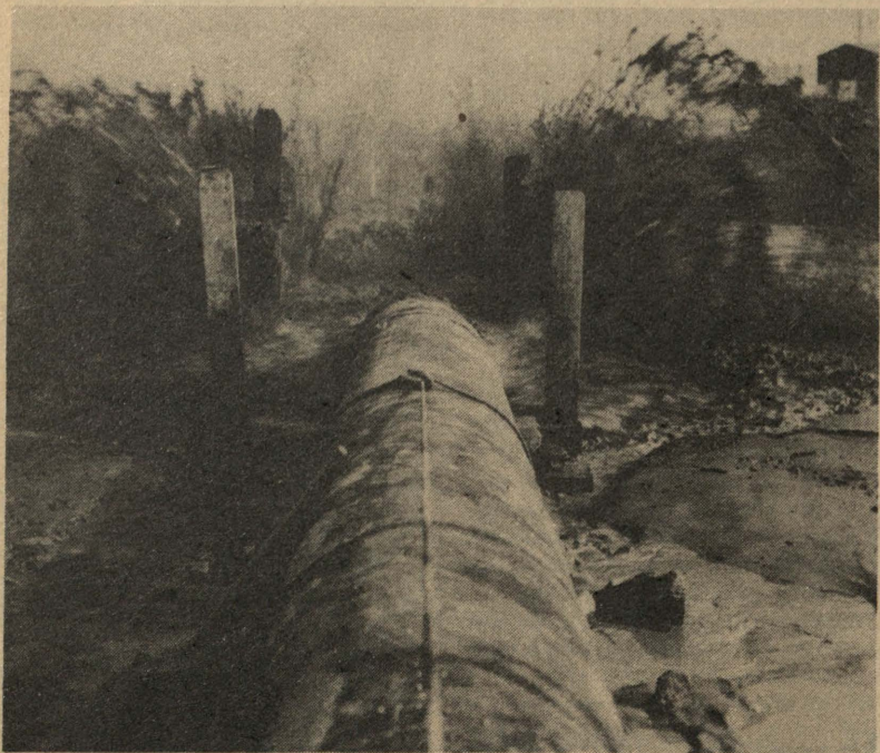
At one time during the dredging the pipe line extended on floats to the north end of the Mock's Bottom parking lot where the force of the pumping operation can be judged by the splash of water and mud coming from the mouth of the pipeline. The pipeline had to be uncoupled every time a vessel went in or out of the Swan Island Outfitting and Repair basin. (Swan Island photos)
