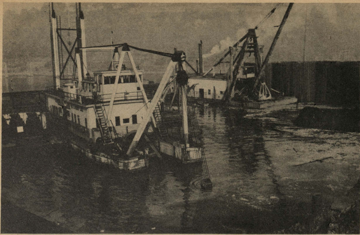
This dredge operates below water with a pipeline, in the center of which is a gadget resembling a huge corkscrew that loosens the earth for the pump to suck through the line. The second dredge at right is the bucket type used to fill many of the cells. The picture was taken shortly after dredging commenced.
