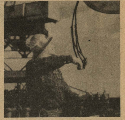
Lower As the load nears the ground, Vancouver Rigger Marvin Bragee signals the operator to lower the load—gently.
