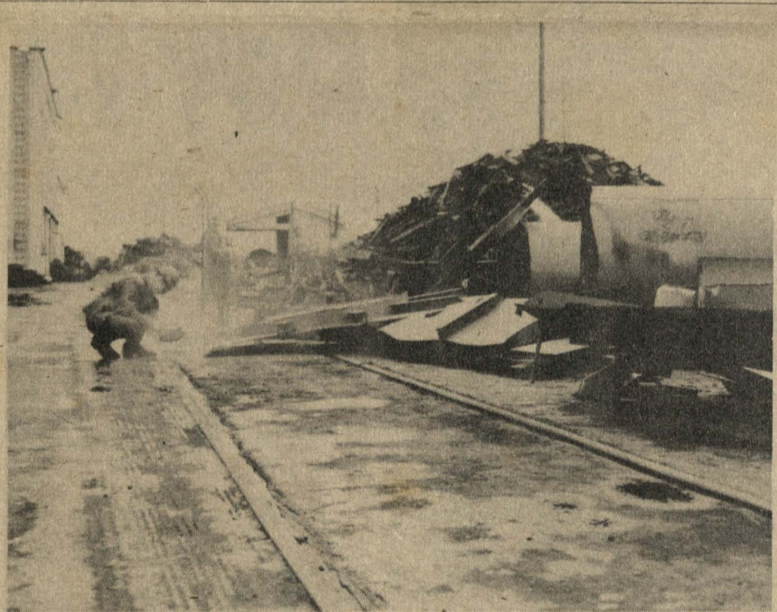
Smelter Food Salvage burners Ray Crowell, on the gun tub, and Vic Haffey, on the ground, are cutting up steel at Swan in tanker gun tubs and other minor sections so the metal can be handled for shipping to smelters.
